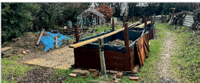
Woody's Lodge Peace Garden (mid-project) Showing recently installed raised planters and paving slabs that, once complete will give better wheelchair access to the garden.
